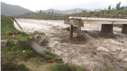
San Vicente Bridge Washed Out
